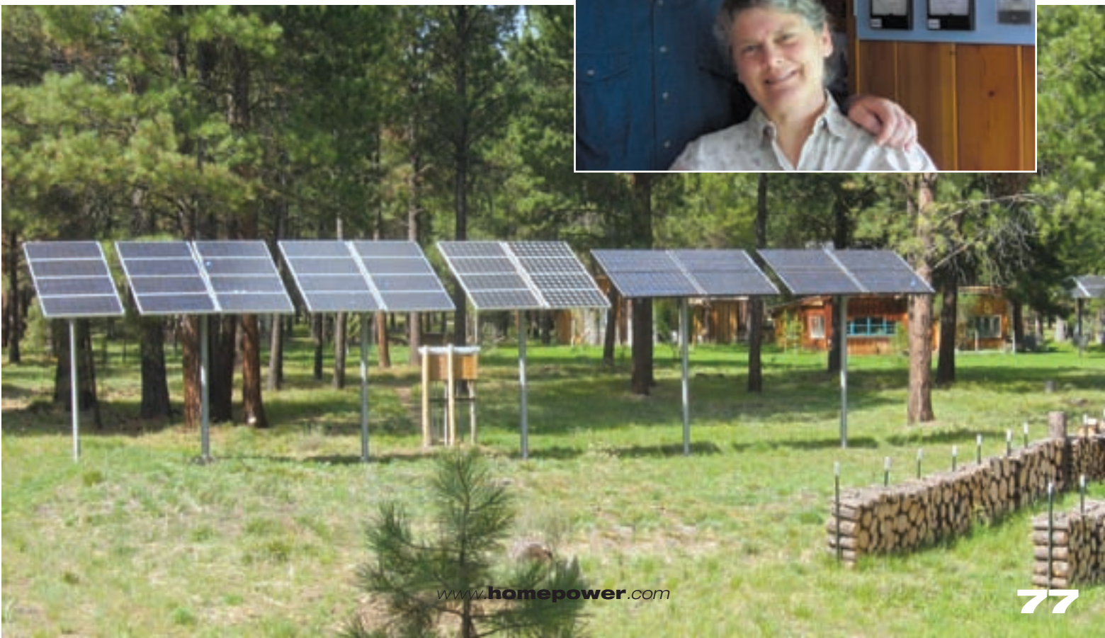
The Barkers’ pole-mounted PV system has grown from one 32-watt module in 1979 to a 5,000-watt array using 44 modules today.
