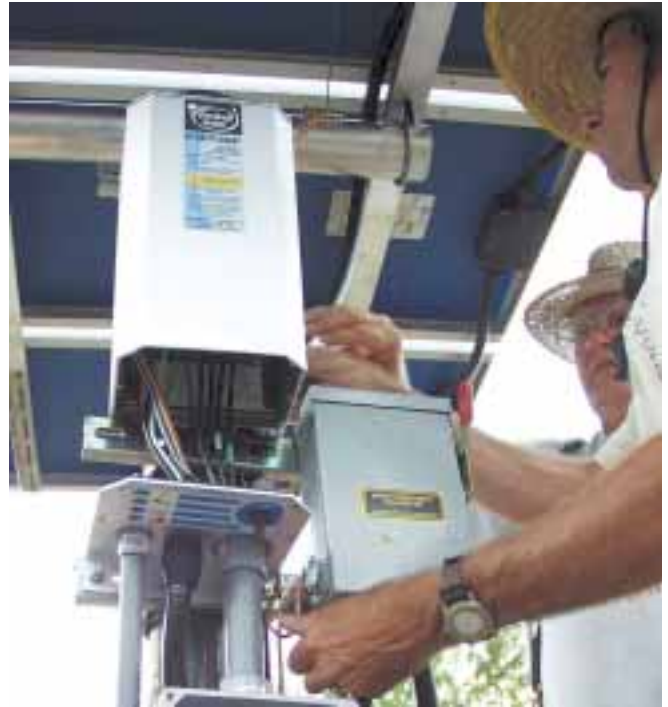
The pump controller wired.
