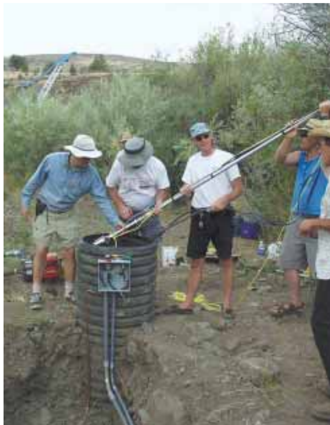
Windy Dankoff (far left) advises the crew on lowering the pump in—the well is only 20 feet (6 m) deep.
