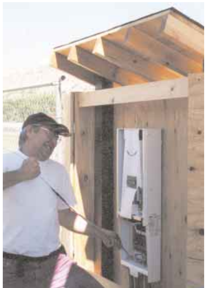
Top: Attaching the home runs to the array. Bottom: Pulling the home runs through the conduit and into the inverter.
