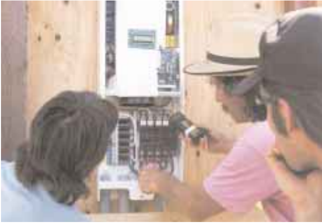
Measuring PV array voltages before putting the Sun Tie inverter online.
