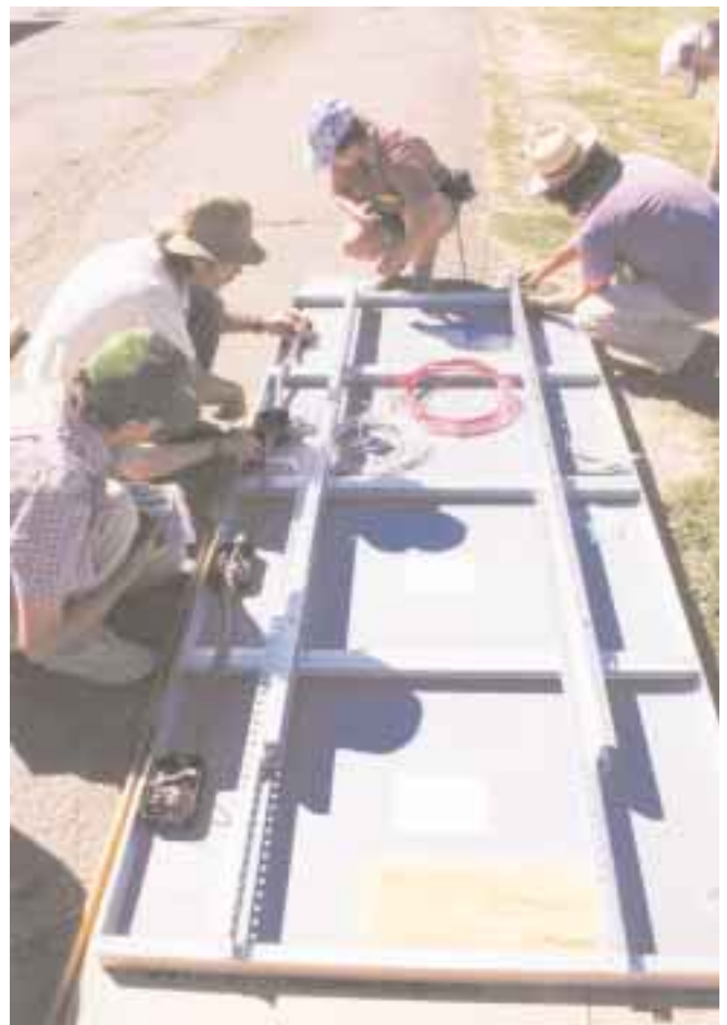
Top: Hey, the rack is too small for these PVs.... Bottom: A successful rack klüge using steel angle iron.
