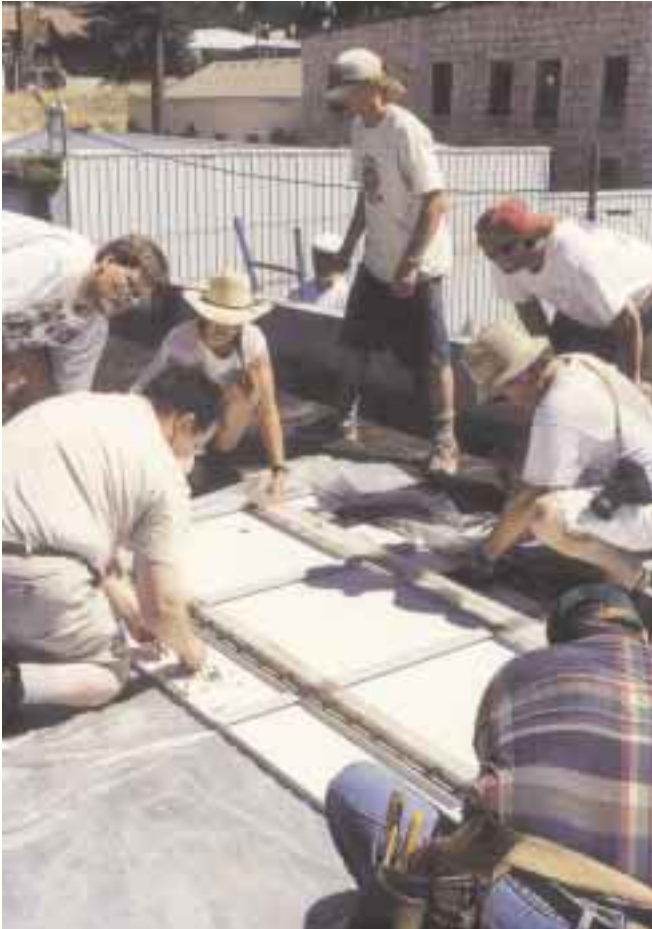
Rack 'em and stack 'em—Sixteen students learned about photovoltaics while helping to install the system.
