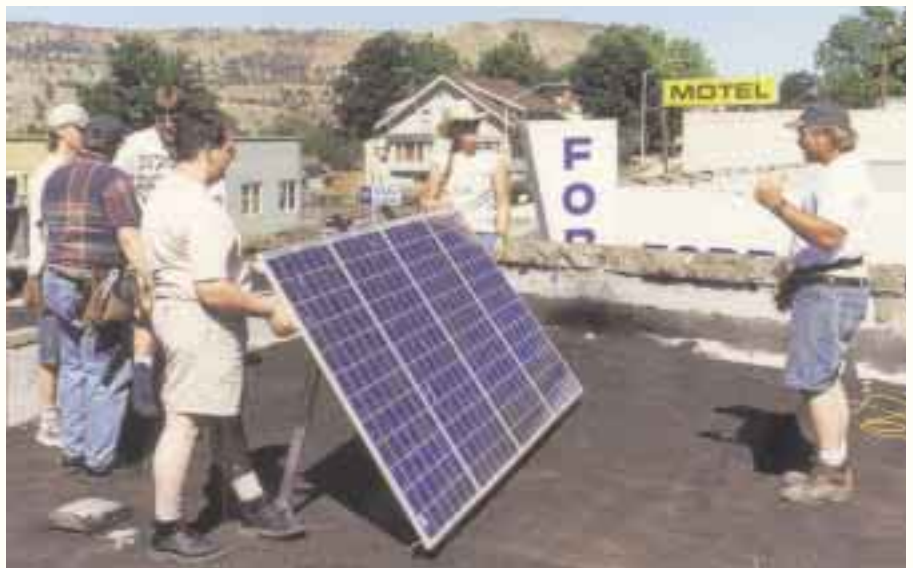
Four Photowatt PW1000, 90 watt modules, in the relentless Eastern Oregon sun, should easily meet the office loads .
